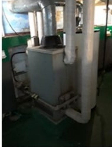
Attic unit with water tank
