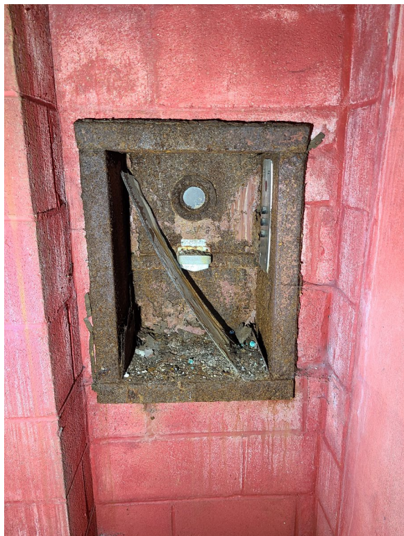
Figure 14. Door to the dumbwaiter in the basement, looking south. Source: Loughlin, June 2023.
