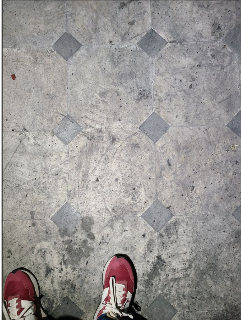
Figure 13. Detail of the Italian marble flooring in the bank lobby. Source: Loughlin, 2023.
