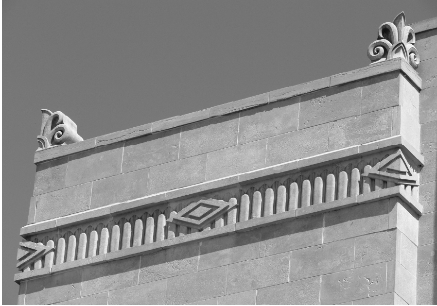
Figure H Detail of frieze, parapet and anthemia on south (Harrison Street) façade.
