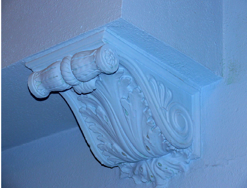
Figure M Detail of Scrolled Bracket supporting the Balcony in the Blue Lodge.
