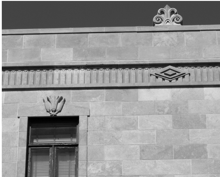
Figure J Detail of window surround, frieze and parapet on east (High Street) façade.
