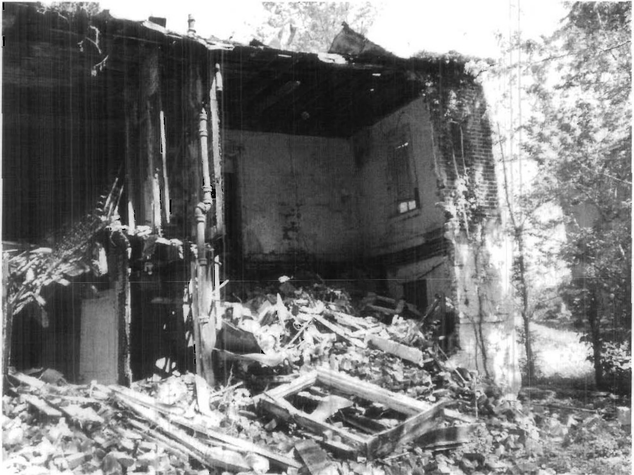
May 7, 2003; collapse of the rear addition
