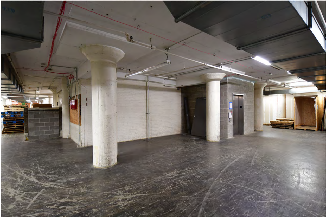
Figure 32. Northwest corner of the second floor of the 1946 addition, looking southeast. Source: Brad Finch, November 2022 (F32 on Photo Map 3).
