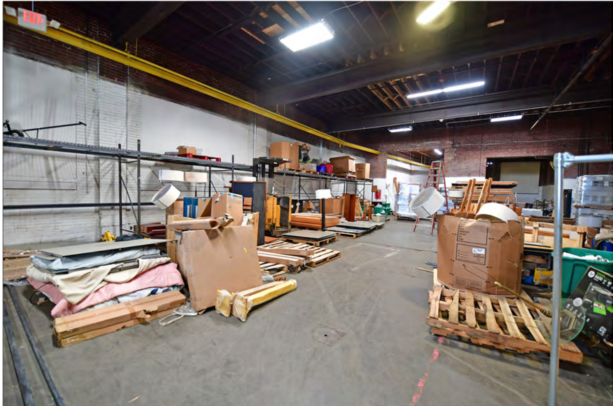
Figure 17. South loading bay addition, looking WSW. Source: Brad Finch, November 2022 (F12 on Photo Map 2).
