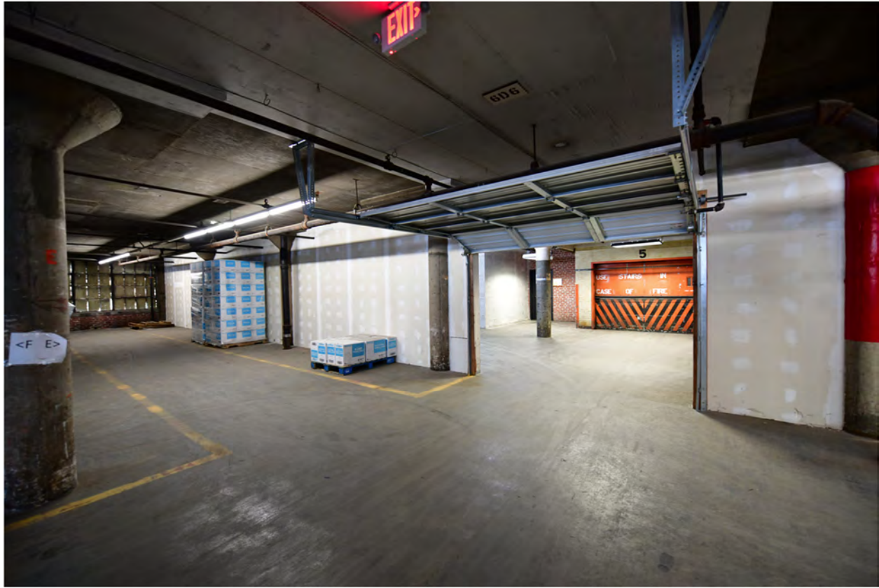
Figure 38. Sixth floor of 1946 addition, looking northwest. Source: Brad Finch, November 2022 (F38 on Photo Map 7).
