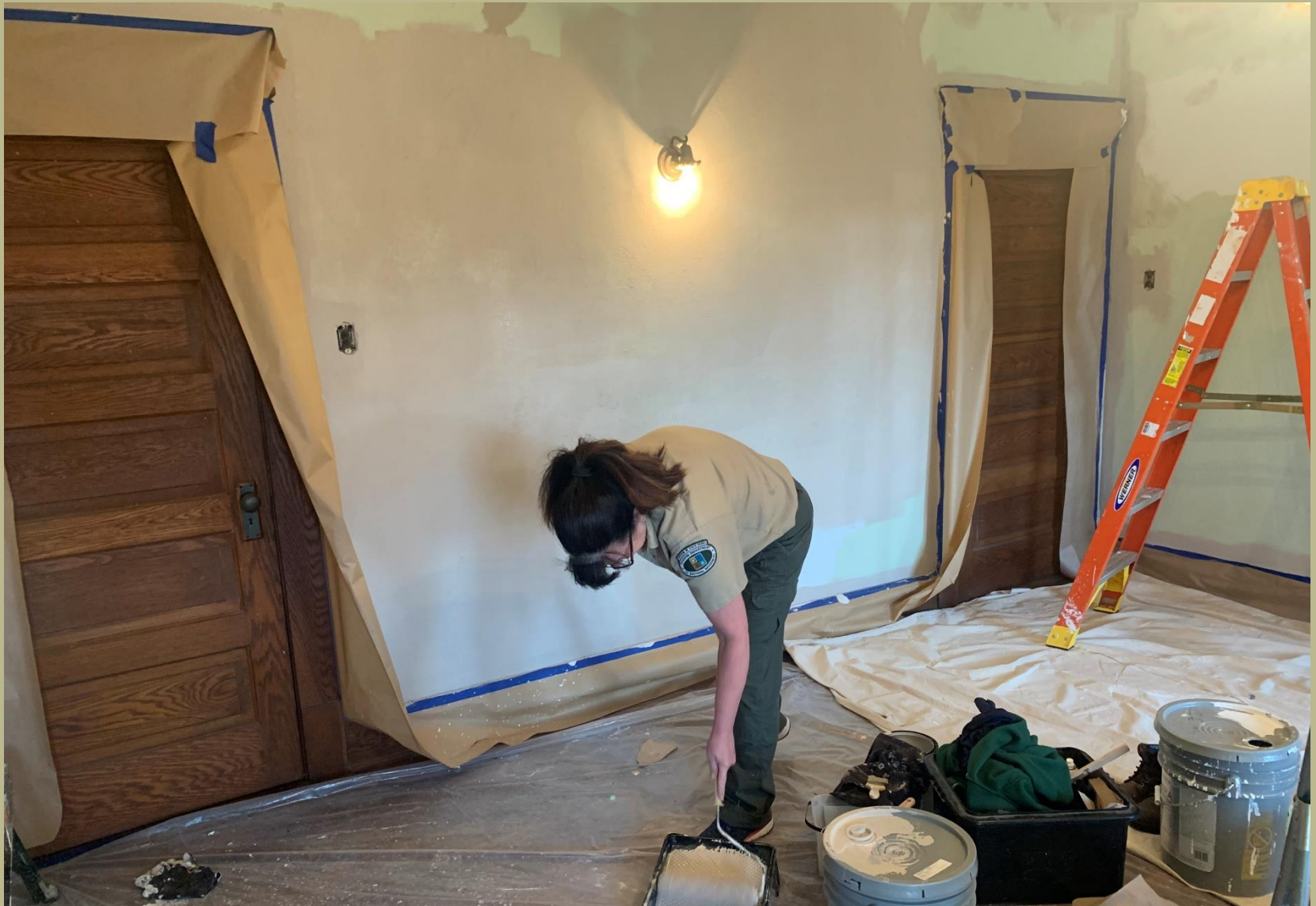
Terry performing plaster and paint repairs in the third phase dining room.
