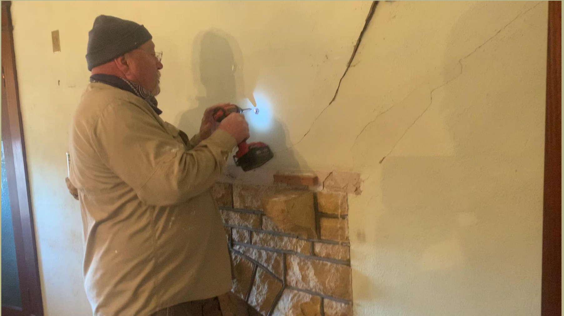
Jeff performing plaster and paint repairs in the third phase dining room.
